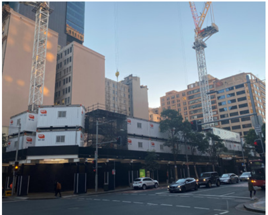
Located in the heart of the city, these Site Sheds provide a range of dedicated spaces
