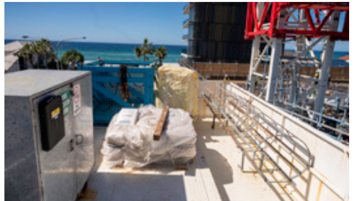
Overhead crane storage for all that extra stuff you need to store
